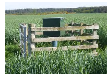
Purpose built borehole
