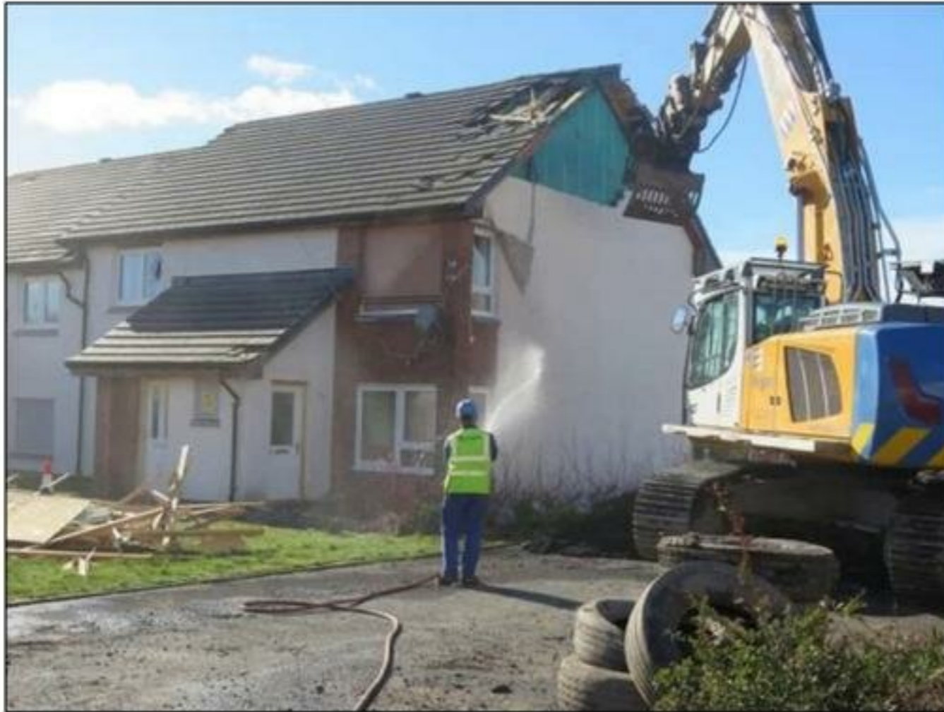
Carbon dioxide ingress – Gorebridge, Midlothian
